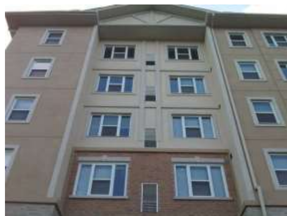
An integrated vent system results in a more attractive and clean building elevation (Waterloo).
