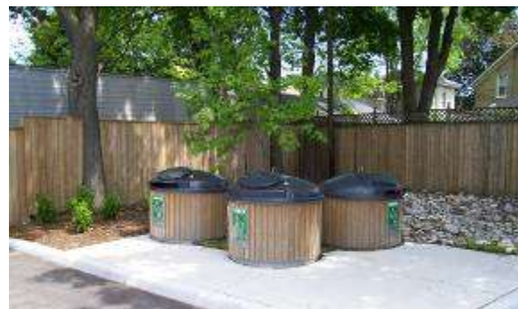
Below grade garbage collection systems, also known as deep well garbage system, provide a compatible alternative to indoor storage location (Kitchener).
